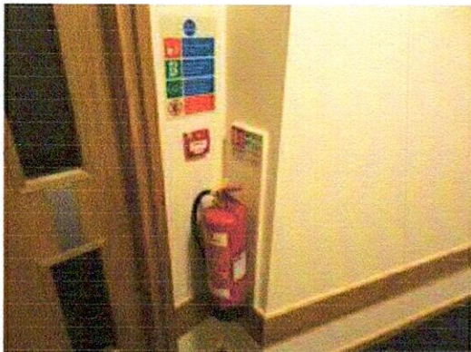
Accessible Fire Extinguisher
